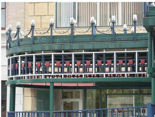
DIFFICULT TO MAINTAIN SURFACES
