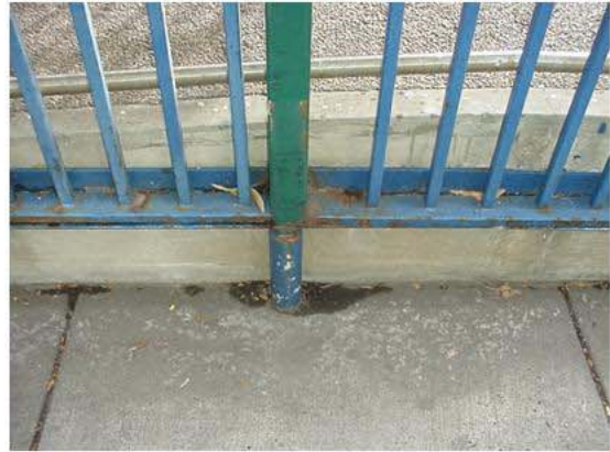
CORRODED STRUCTURAL MEMBERS
