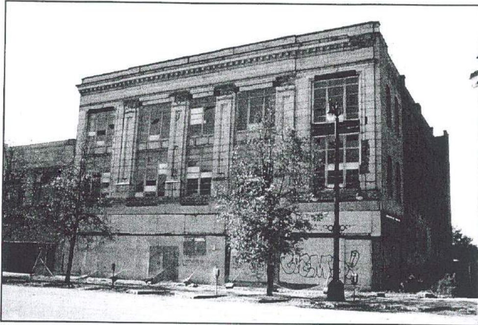
Figure 29. Deteriorated building at 758 Main Street (PCI 2001).
