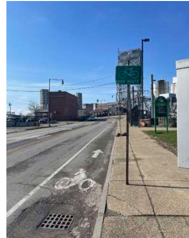
DETERIORATED BICYCLE LANES
