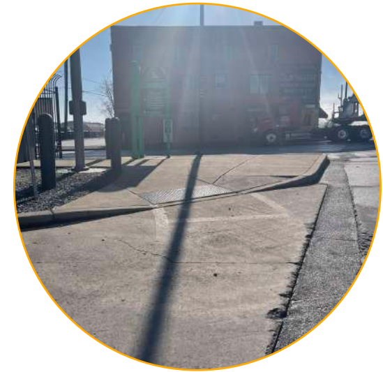
6 Crosswalk striping is almost completely faded out across the NFTA facilities driveway.
