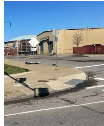
CURB RAMP PAVEMENT FAILURE
