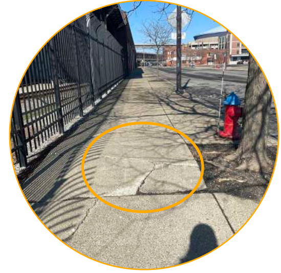
3 Sidewalk heaving due to street tree roots, presenting potential accessibility issues.
