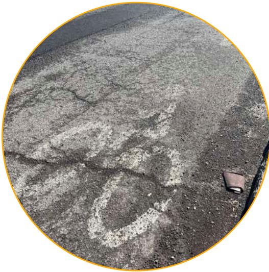
4 Pavement markings for the designated bicycle lanes (as well as lane striping) on South Park Avenue are very faint and hard to discern.
