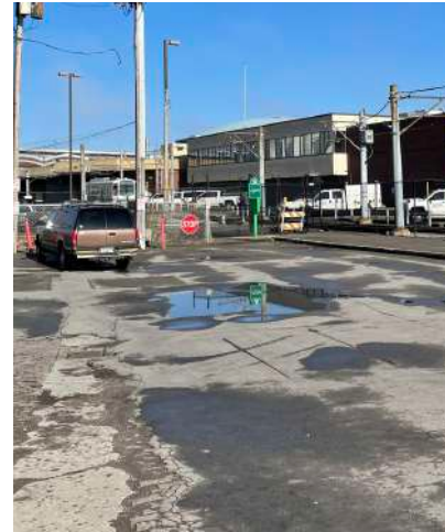
PAVEMENT CONDITION @ GATEWAY
