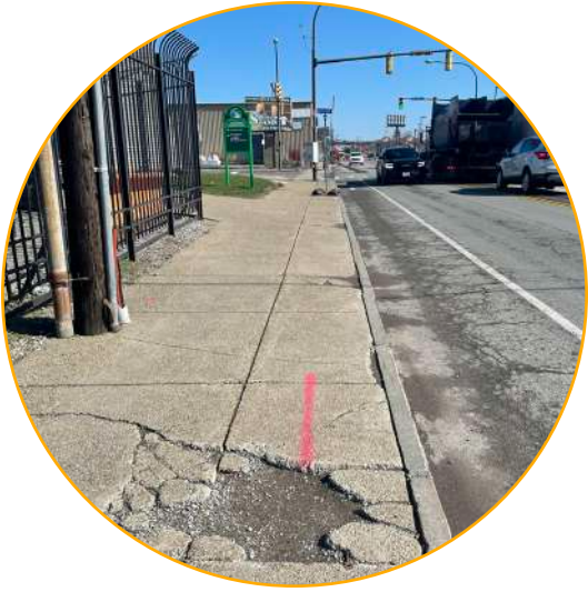
5 The sidewalk is cracked and significant deteriorated in some spots along Michigan Avenue, creating potential hazards for pedestrians.
