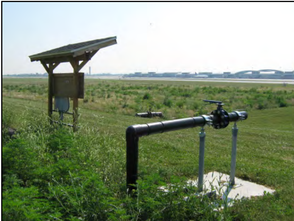
Photograph 12: BNIA's engineered underground wetland for glycol treatment. This photograph shows the #2 cell looking the eastward towards the terminal. (MJ Photo 07/07/10)
